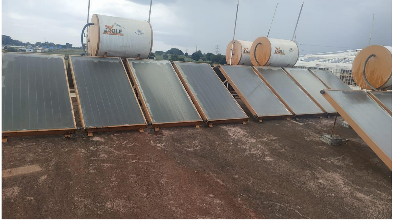
Solar Water Heaters installed on Hostel rooftop
