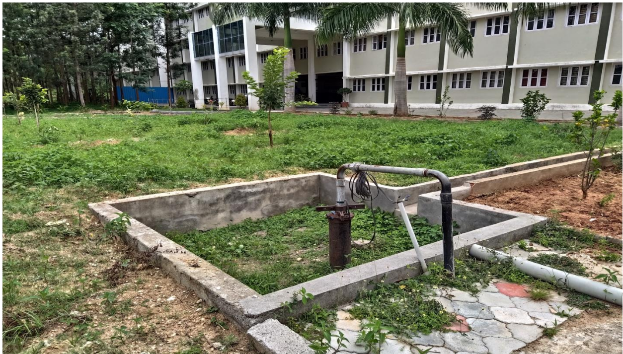
Bore well Recharge Point
